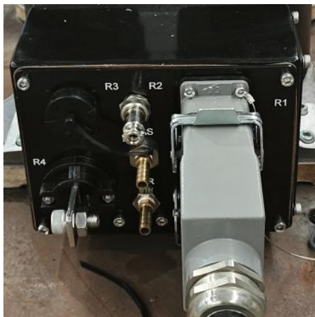
Figure 2.3 Body heavy load connector inspection
